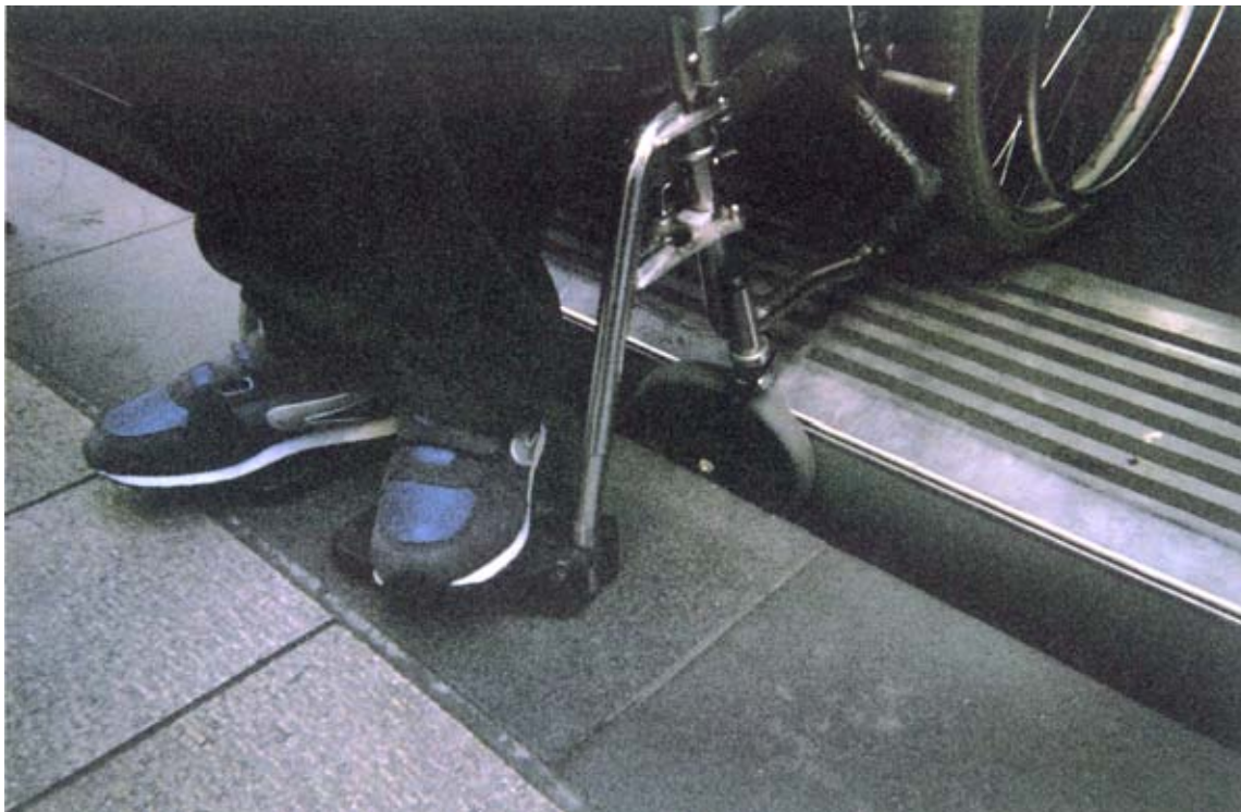
Location of photo: Box Hill Tram Route: Collins St raised platform stop – Melbourne.
